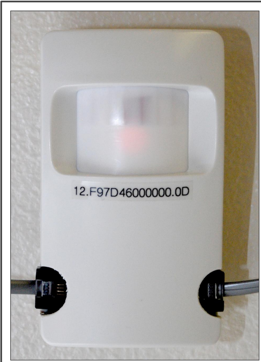
Ceiling-mounted motion sensor from testbed.
